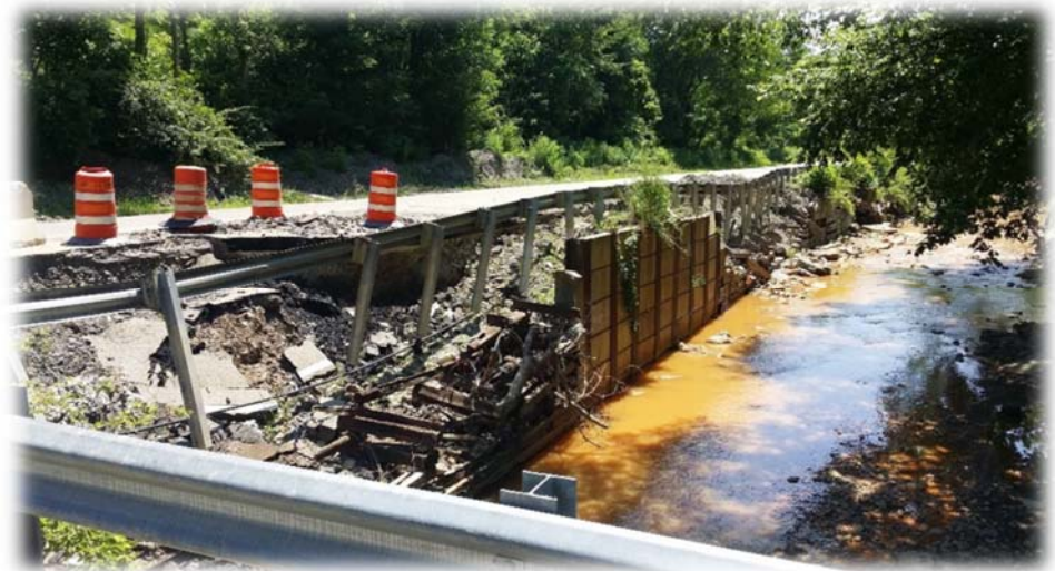
Willow Grove Road Retaining Wall Before Repair
