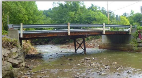
Bridge prior to repair on Wasniak Road Pultney Township T-281
