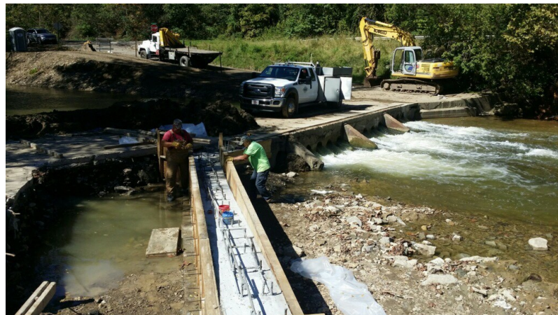
Work is underway to improve the approaches to the Gordon Sub bridge.
