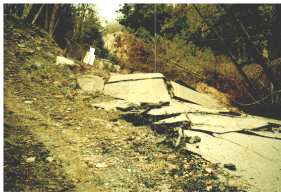
Willow Grove Road Landslide 2000
