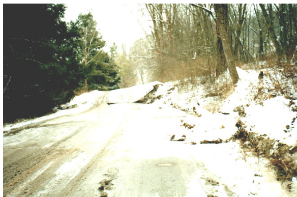
Willow Grove Road Landslide 2000
