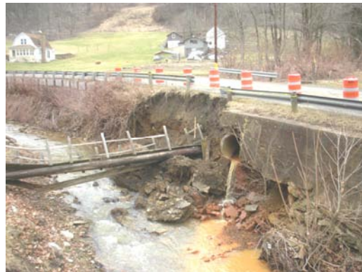
County Road 2 Deep Run slip.
