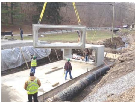
Concrete box culverts were set on the bridge replacement project on Brown's Run the week of March 16th.
