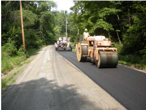
Lash Excavating & Paving working on Co. Rd. 5 Crescent - 250 and at right, Co. Rd. 84, Airport Road.
