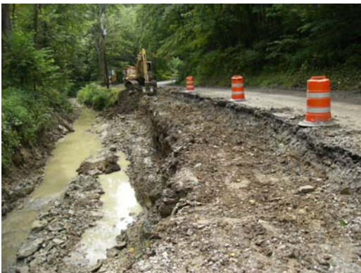
Work began this week on the roadway slip on County Road 5, Glencoe St. Clairsville.
